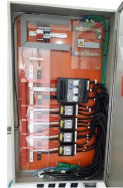
Fig. 8. Internal image of the second inverter switchboard installed on 16/03/2022 at the substation of the 406kWp photovoltaic plant.
