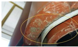
Fig. 12. Dust and coil failure. 406kWp power plant.
