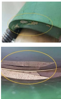
Fig. 14. Faulty resin or surface paint and cracked insulation. 444kWp plant.
