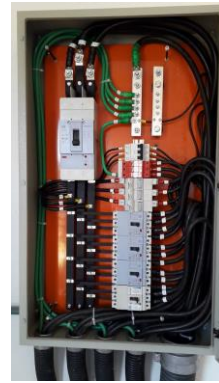
Fig. 7. Internal image of the first inverter switchboard installed on 15/03/2021 at the substation of the 406kWp photovoltaic plant.
