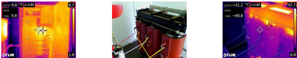
Fig. 9. Thermography of the QGINV on 19/05/2022 at 16h and 30 min in the 406kWp plant. Thermal image of the transformer on the same date and time. The ambient temperature on the same date and time was 12.5°C (at the weather station installed near the substation).
