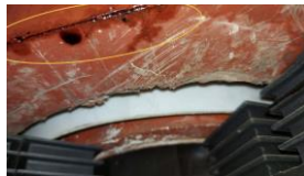
Fig. 13. Crack in the epoxy resin insulation. 406kWp plant.
