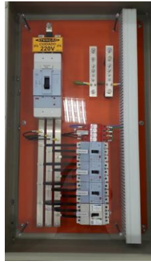
Fig. 6. Internal image of the first inverter control panel.
